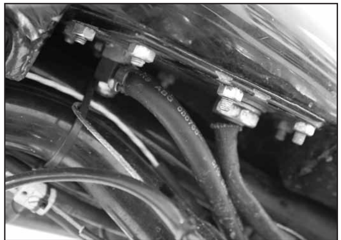
Figure 3: Custom mounting plate at bottom of the tank
